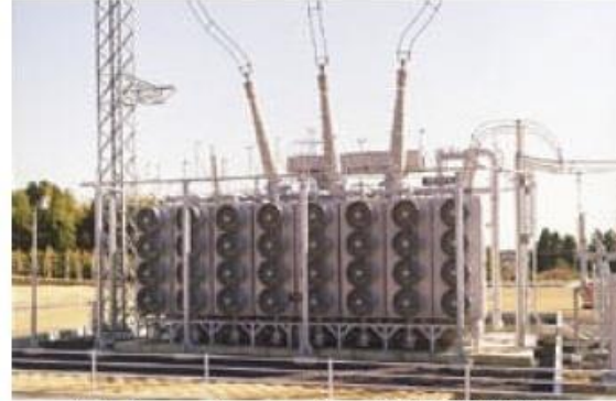
(b) transformator 4500MVA
