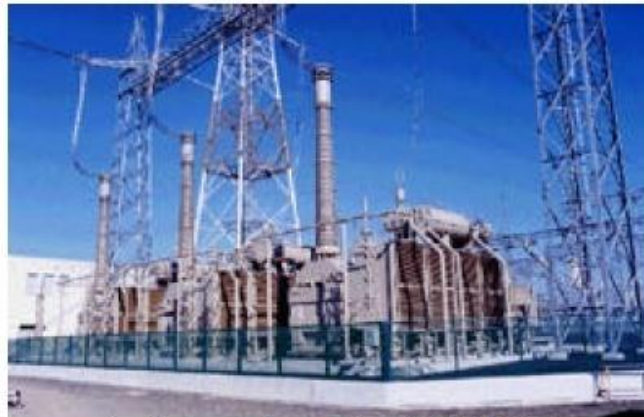
(c) Transformator 1000MVA
